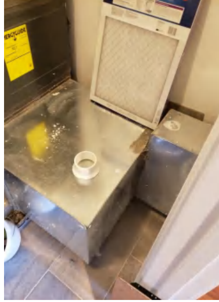
Lower Level Furnace Return Duct
