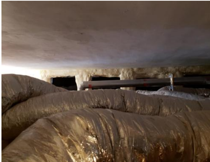
Fireplace Ductwork (Uninsulated sheet metal duct in back)
