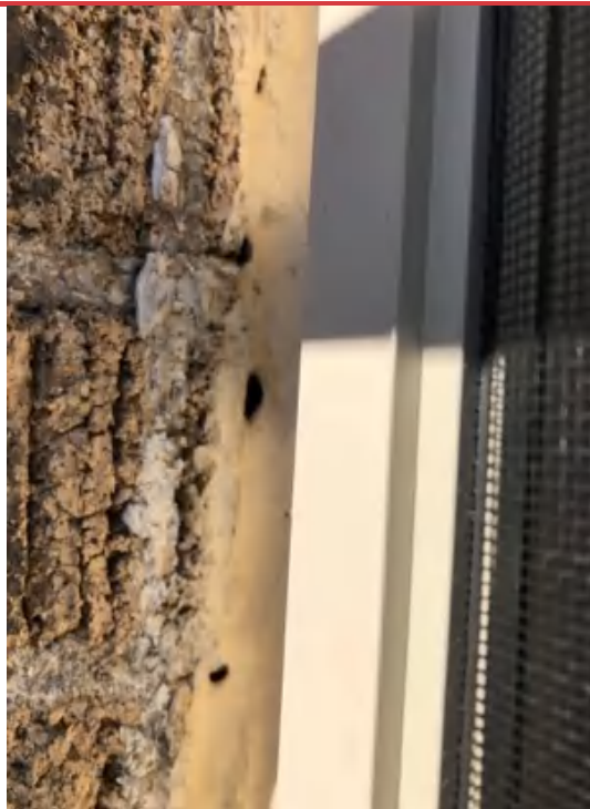
CLOSE UP TO SHOW HOLES Large holes in caulk. Poorly installed.
