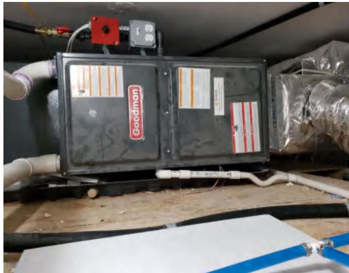
Mid-Level Furnace in Ceiling Space
