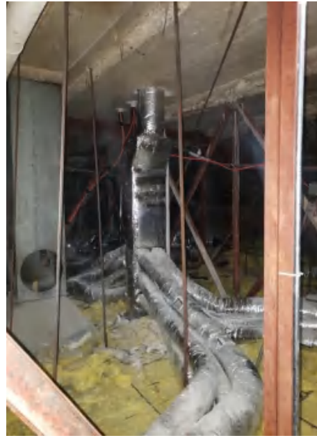
Common Duct to Roof
