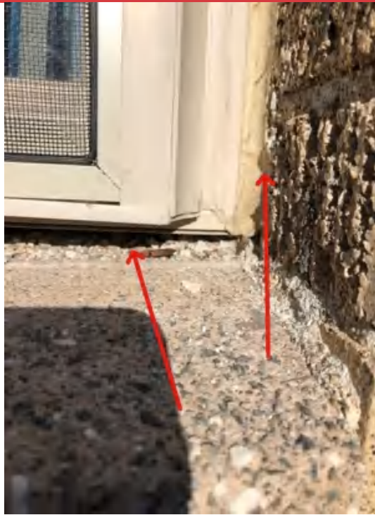
WINDOW AS OF 1/5/21 Completely open and unsealed.
